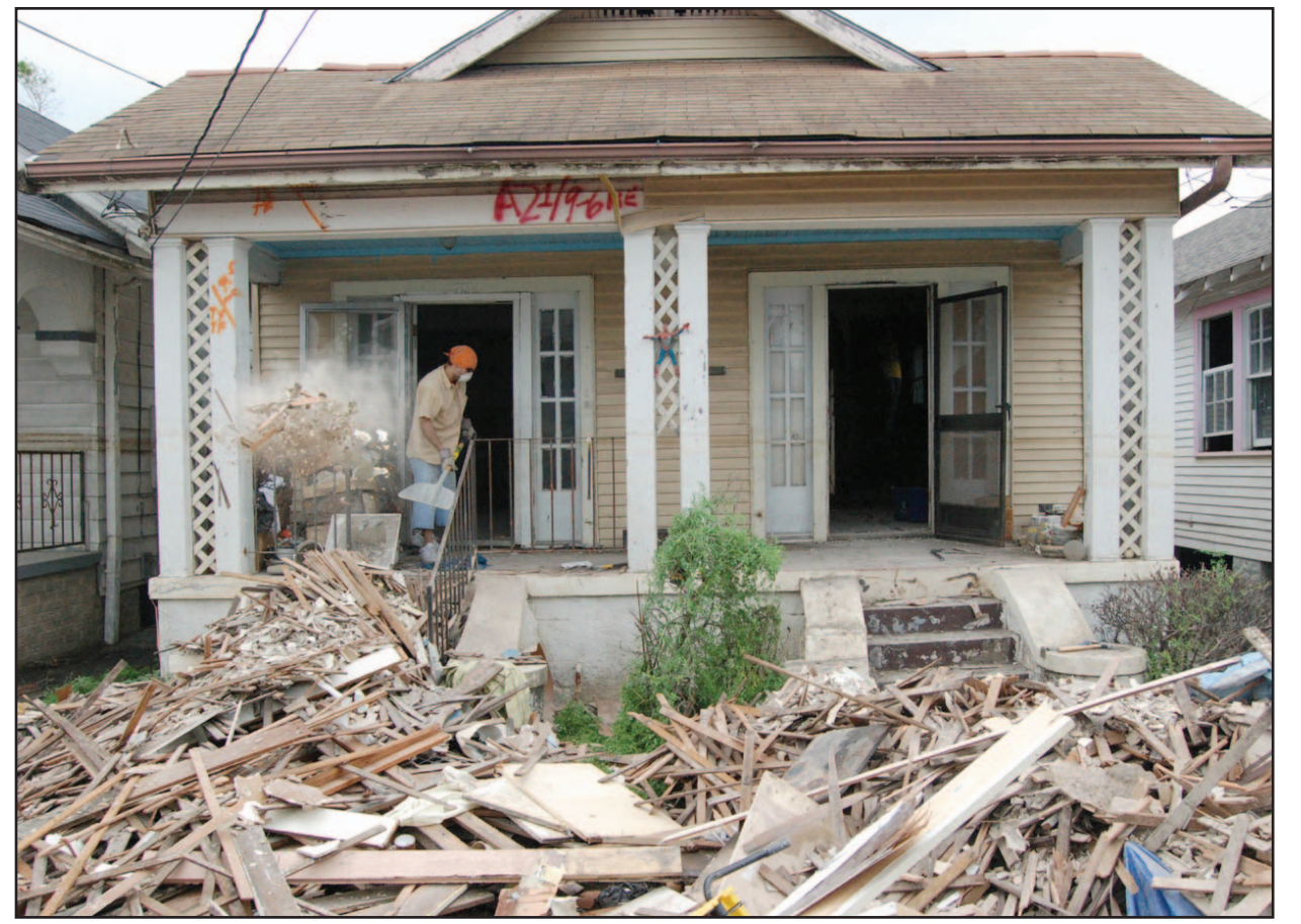
The guts of Lori Marquez's house in the Lower Ninth Ward of New Orleans fills the front lawn as Sam Glover of UMass Dartmouth shovels another pile of debris.
