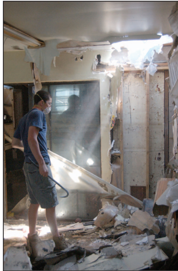
Above, sunlight streams through holes in the Mitchell's house as Frank Pearson rips down the moldy walls.
